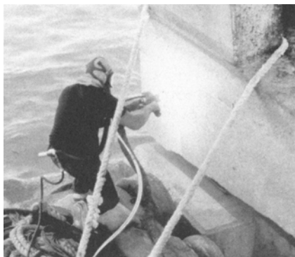
Zinc thermal spraying process being applied on the Seven Mile Bridge in Key West, Florida, 1992.
